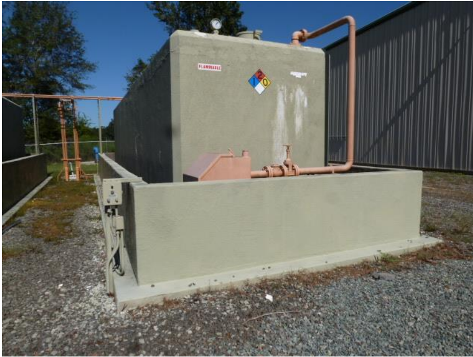
Photograph I – Diesel Storage Tank Efflorescence
