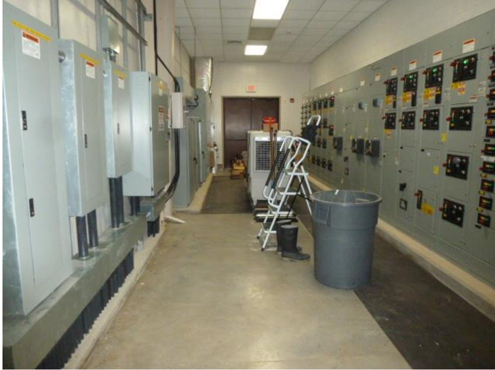
Photograph U –Chemical Building Electrical Room
