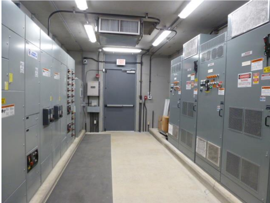
Photograph G – Pump Station Electrical Room
