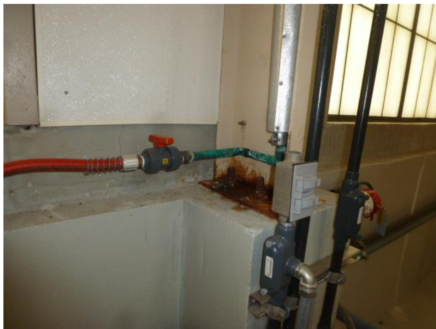
Photograph T –Chemical Building Corroding Column
