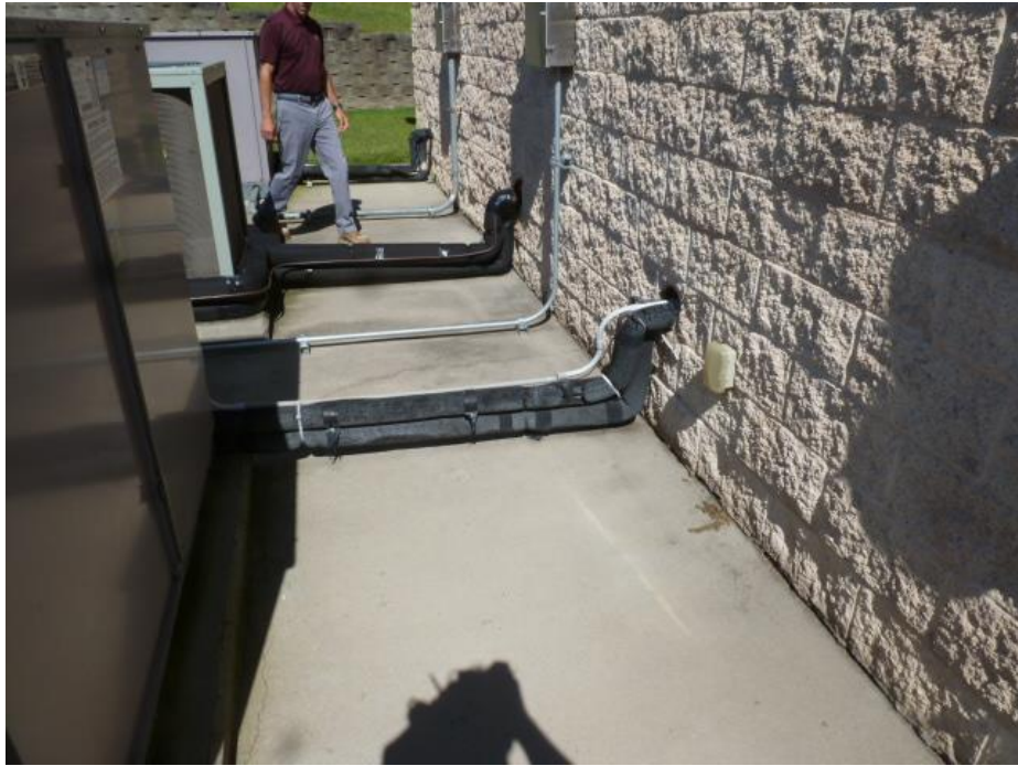
Photograph G – Failing HVAC Coolant Insulation
