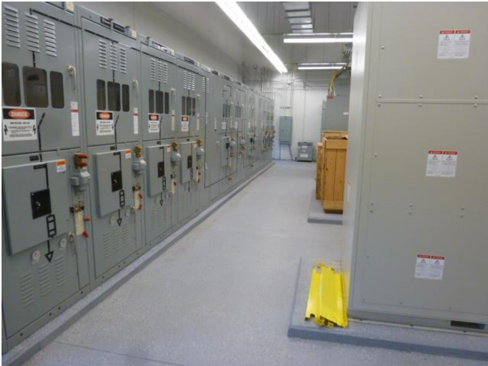
Photograph D –Electrical Room
