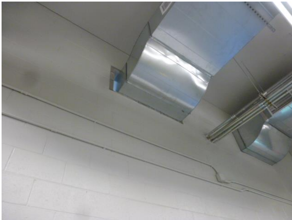
Photograph F -HVAC Penetration into Electrical Room
