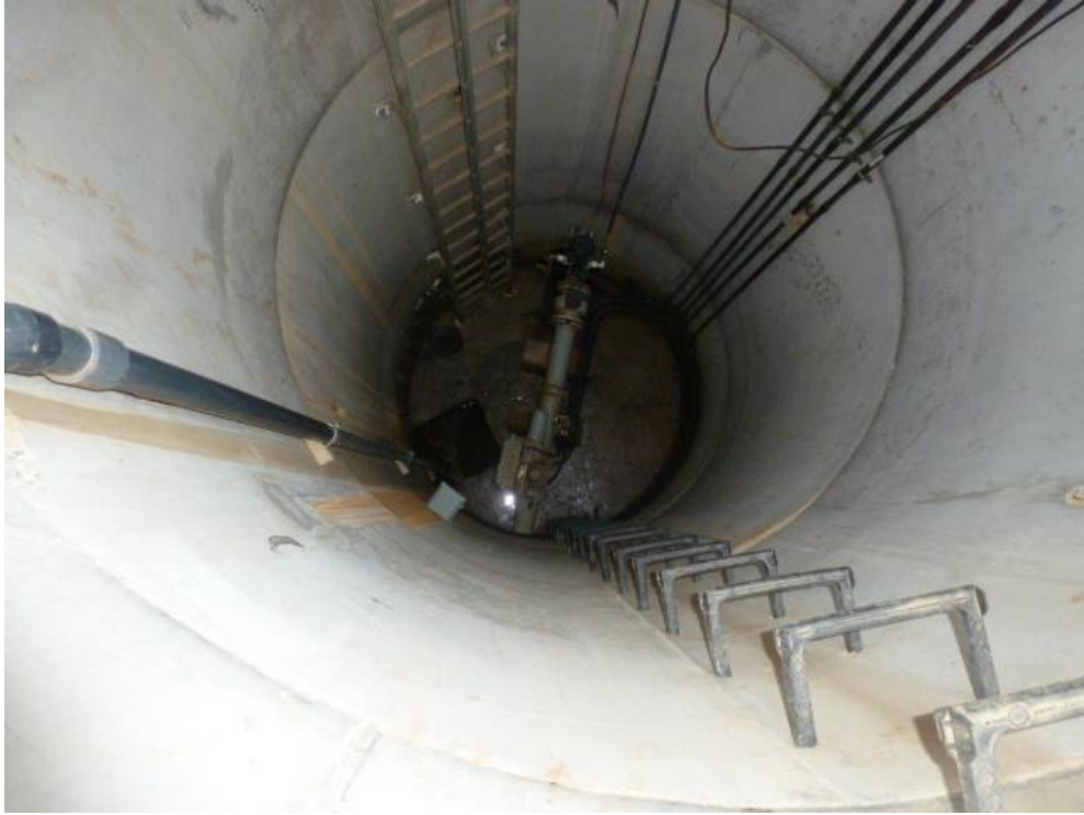
Photograph W –NPDES Meter Vault
