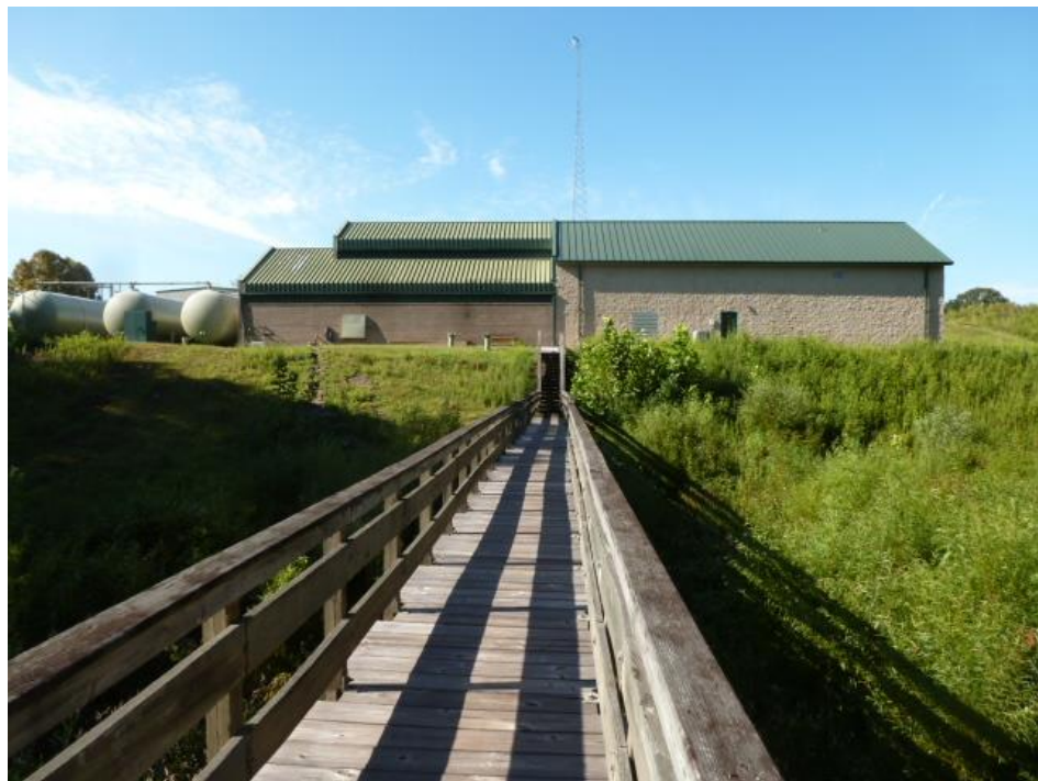
Photograph P – Distressed Air Backwash Pier Access
