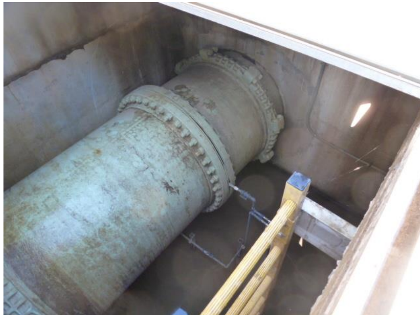
Photograph H – Pump Station Effluent Flow Meter
