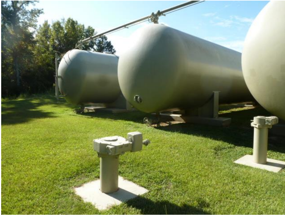
Photograph M- Surge Tank Valves Paint Peeling
