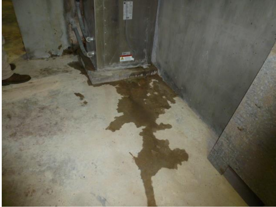
Photograph O – Filter Gallery Leak
