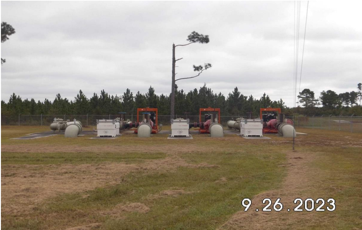
Photograph S – Interim Booster Station
