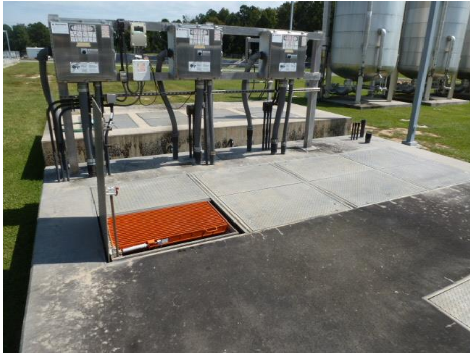
Photograph P – Transfer Pump Station
