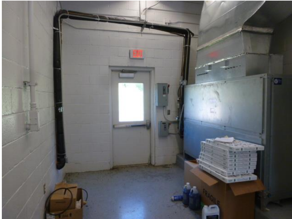
Photograph E -HVAC Room
