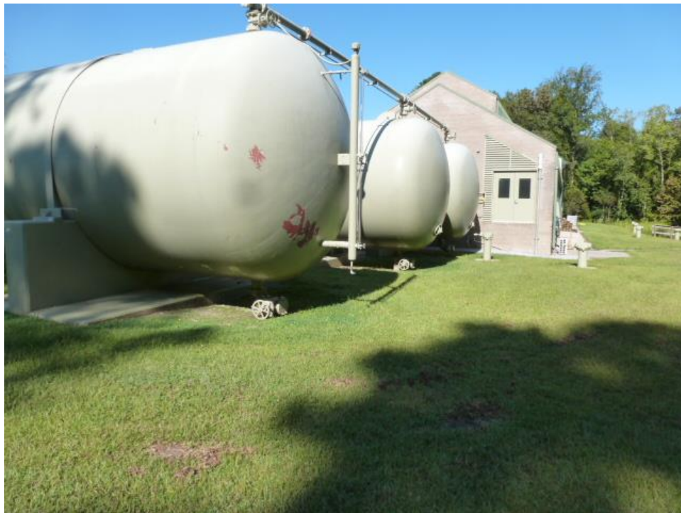
Photograph L- Surge Tank 3 Paint Peeling
