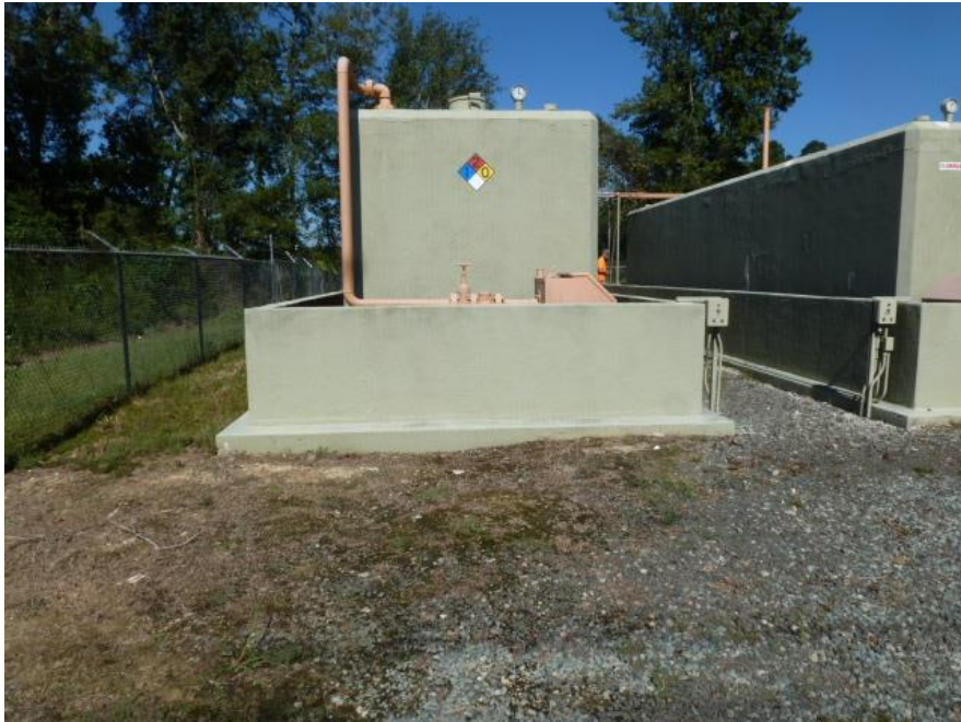
Photograph J – Diesel Tank with Failed Leak Sensor Panel
