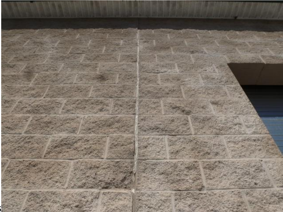
Photograph C – Existing Crack in Electrical Building Wall
