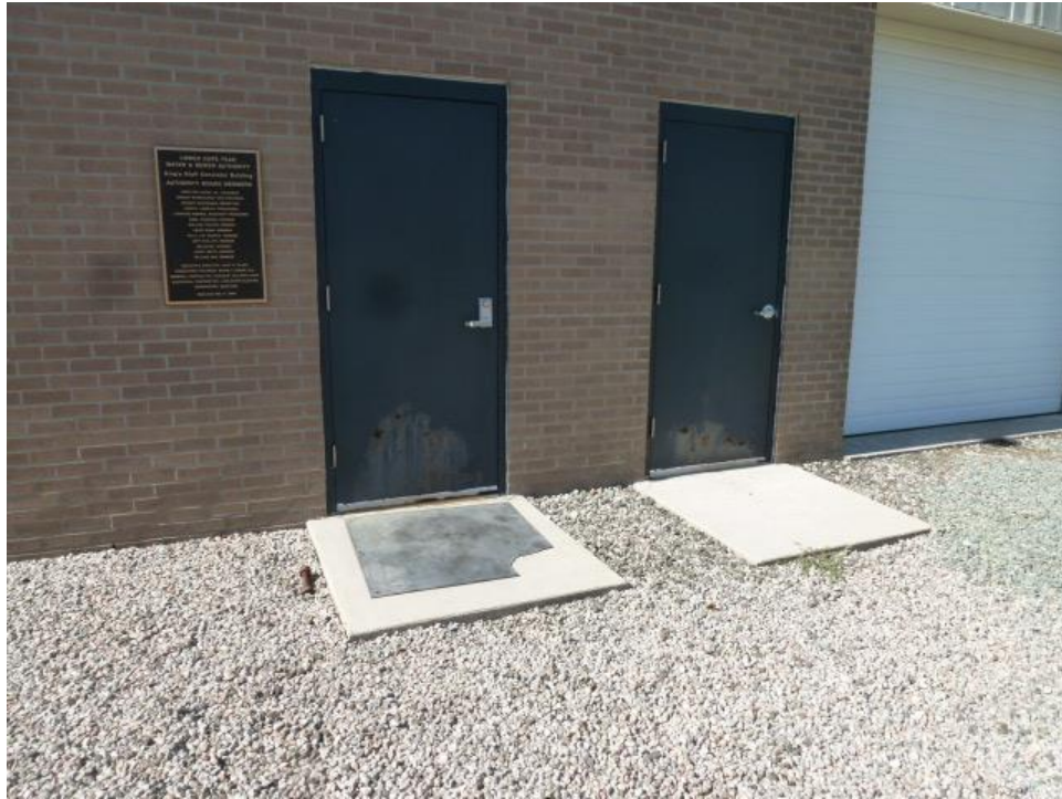
Photograph Q –Generator Building Corroded Doors
