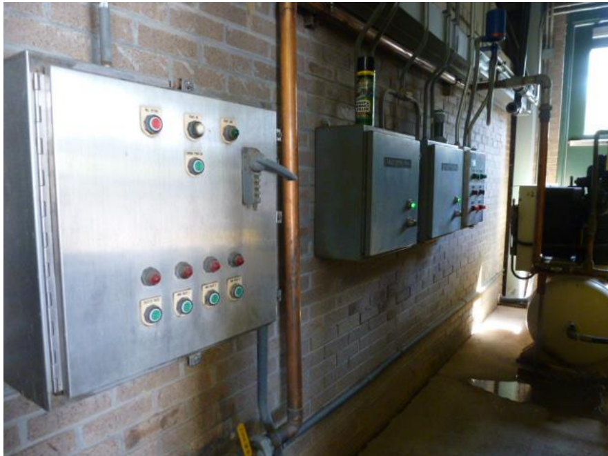
Photograph N- Surge Tank Control Panels
