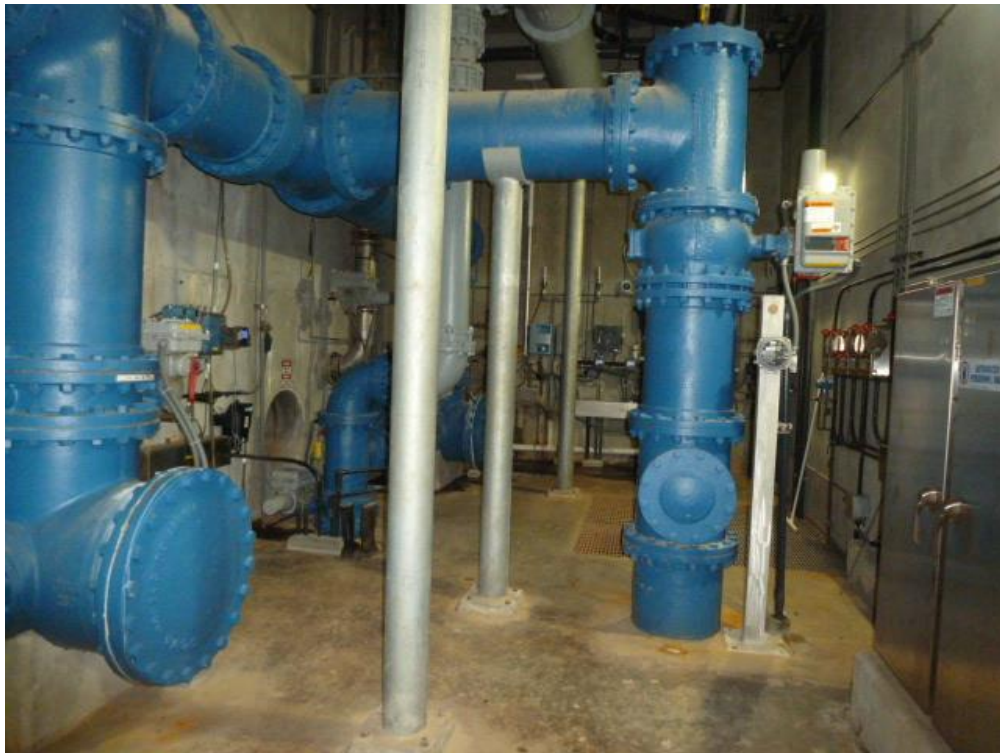
Photograph N – Filter Gallery
