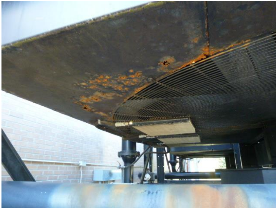
Photograph R – Corroded Radiator Fan Shroud
