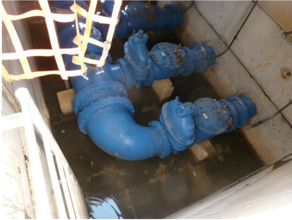
Photograph Q – Transfer Pump Station Valve Vault
