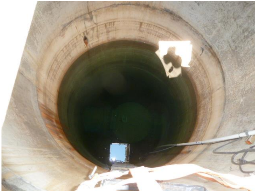
Photograph R – Transfer Pumps Station Check Valve Vault
