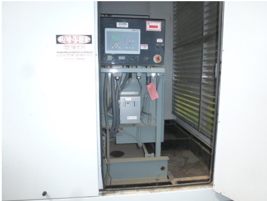
Photograph H – Influent Pump Station Generator Enclosure
