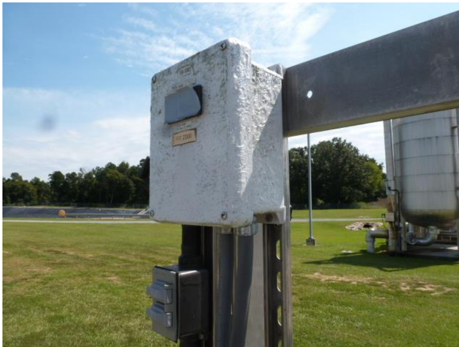
Photograph L – Influent Flow Meter Vault Instrument Display
