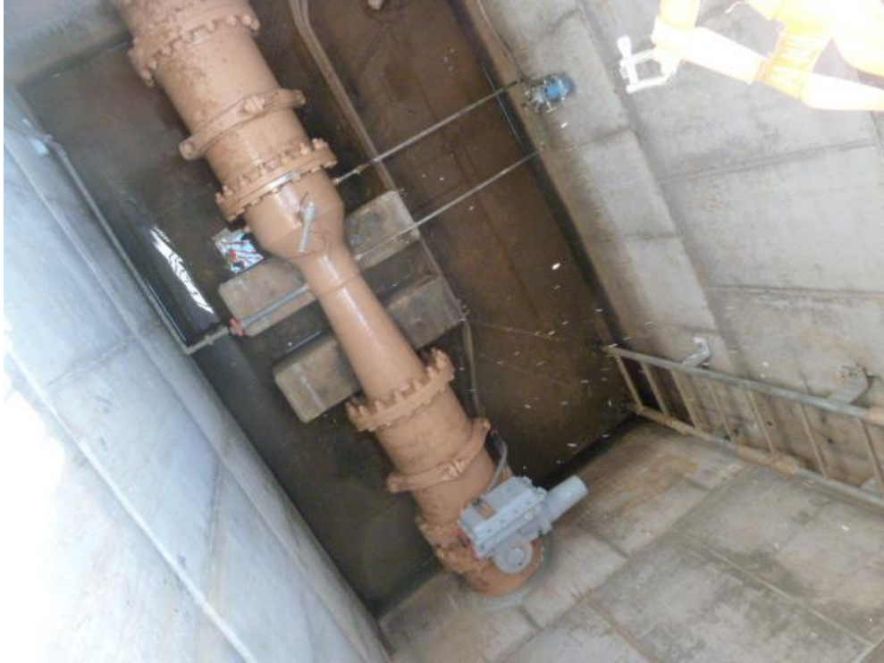
Photograph K -Influent Flow Meter Vault
