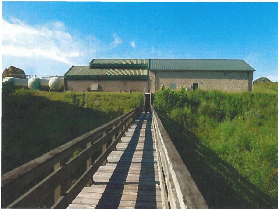
Photograph P – Distressed Air Backwash Pier Access
