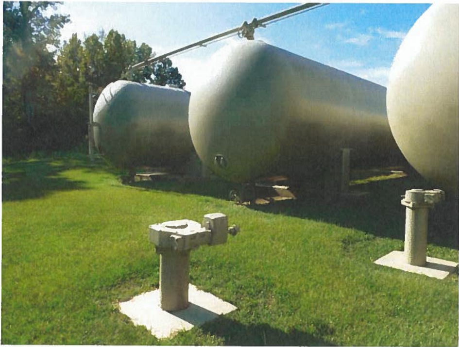
Photograph M- Surge Tank Valves Paint Peeling
