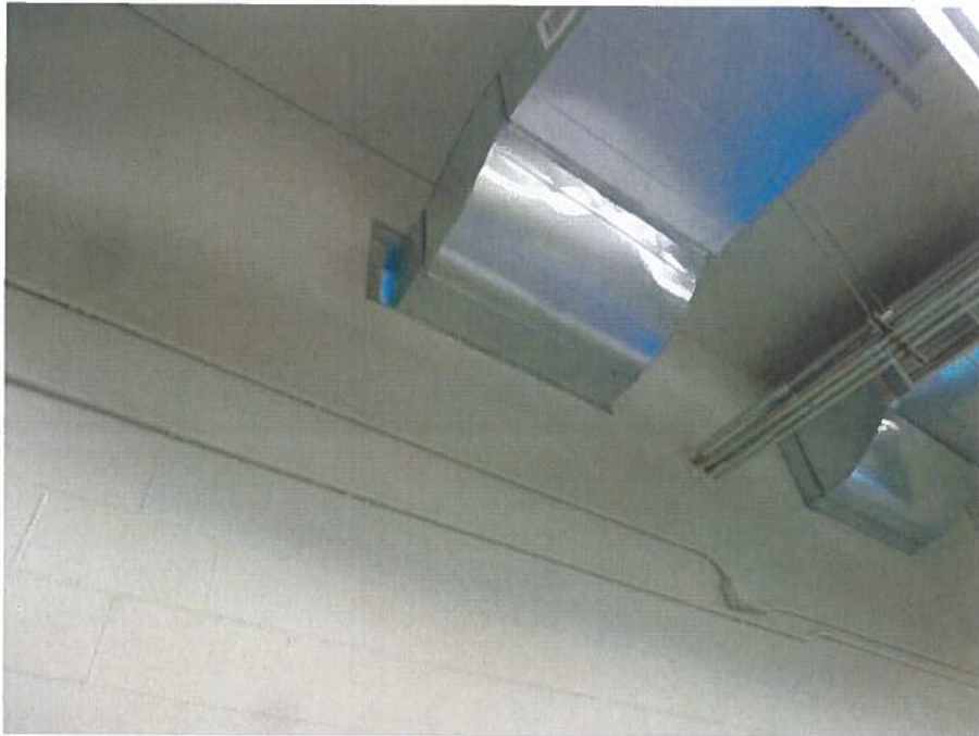
Photograph F -HVAC Penetration into Electrical Room
