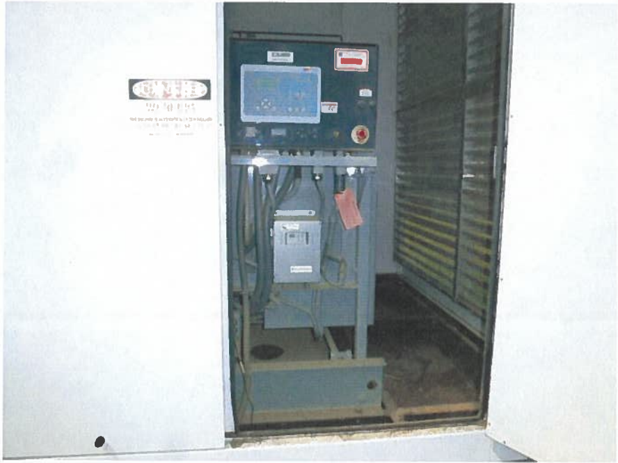
Photograph H – Influent Pump Station Generator Enclosure
