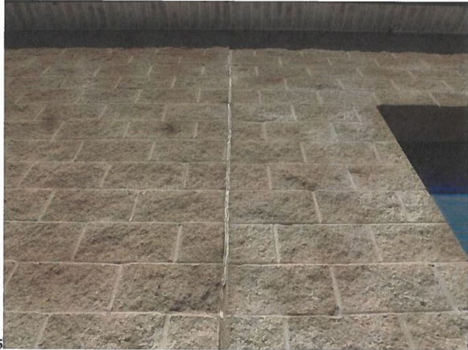
Photograph C – Existing Crack in Electrical Building Wall
