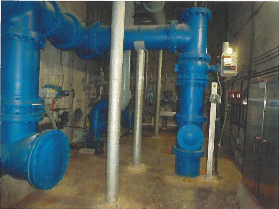
Photograph N – Filter Gallery
