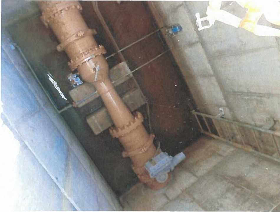
Photograph K -Influent Flow Meter Vault
