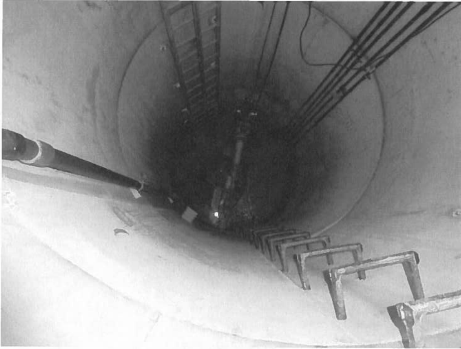
Photograph W –NPDES Meter Vault
