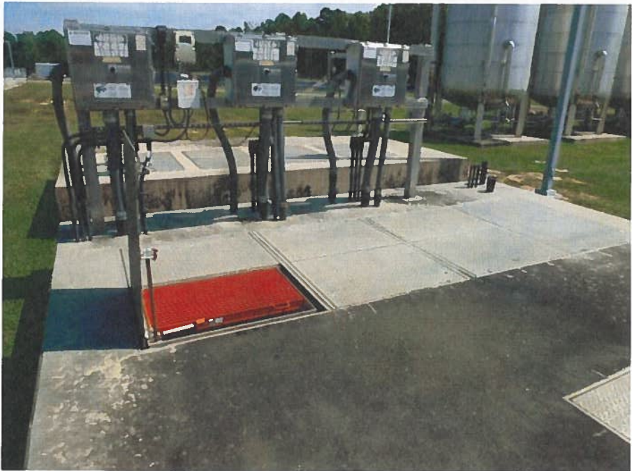
Photograph P – Transfer Pump Station
