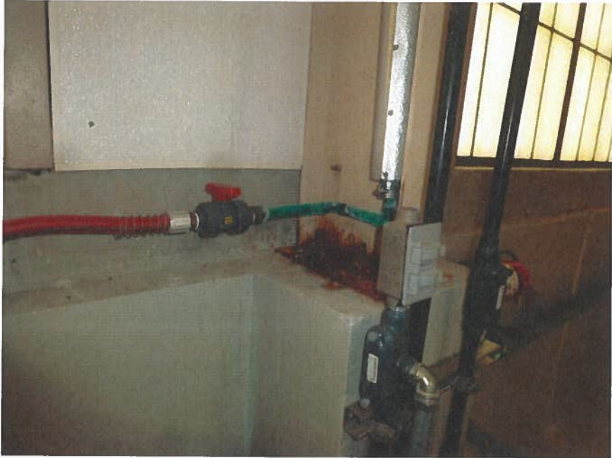
Photograph T –Chemical Building Corroding Column
