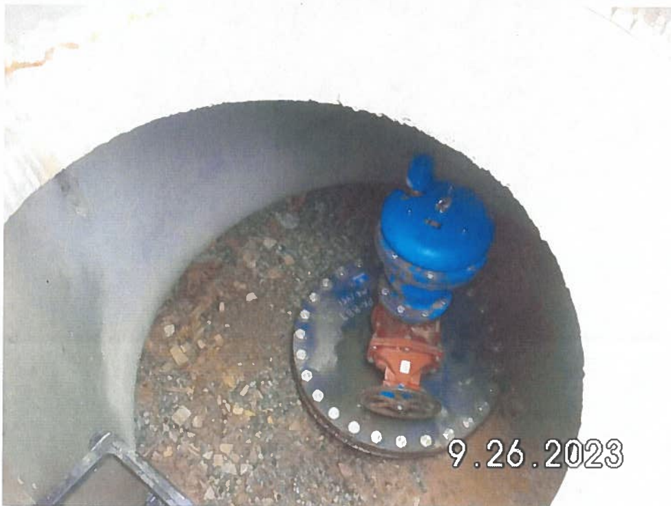
Photograph DD – Old ARV on 48" RWM and New ARV on 54" RWM
