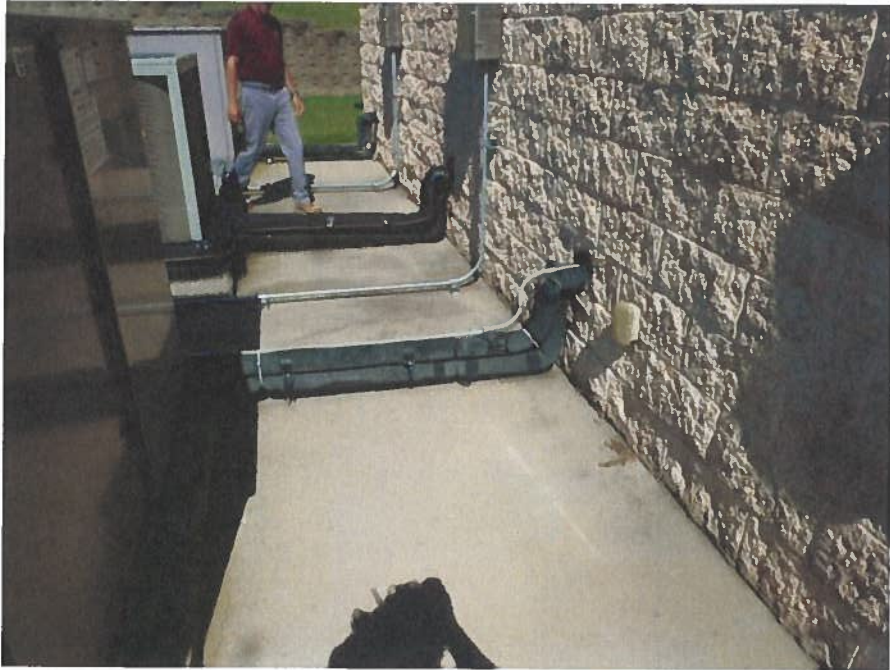
Photograph G – Failing HVAC Coolant Insulation
