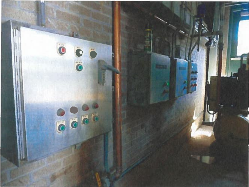
Photograph N- Surge Tank Control Panels
