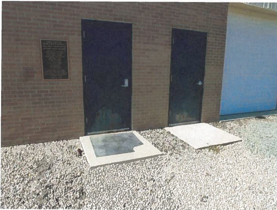
Photograph Q –Generator Building Corroded Doors
