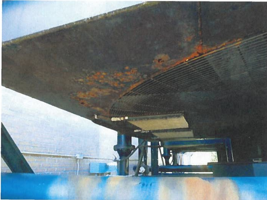
Photograph R – Corroded Radiator Fan Shroud
