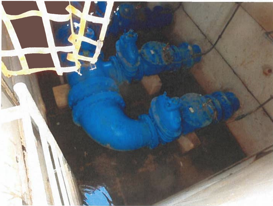
Photograph Q – Transfer Pump Station Valve Vault
