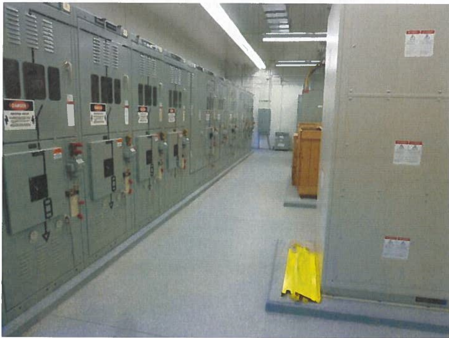
Photograph D – Electrical Room
