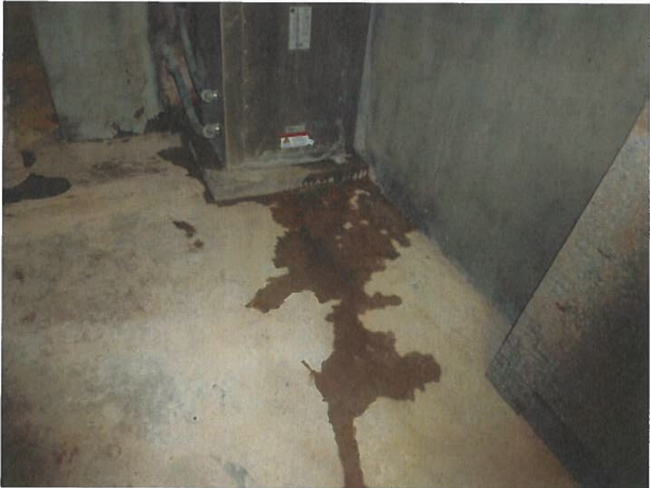
Photograph O – Filter Gallery Leak
