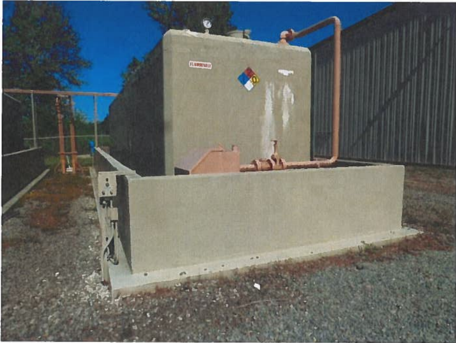
Photograph I – Diesel Storage Tank Efflorescence
