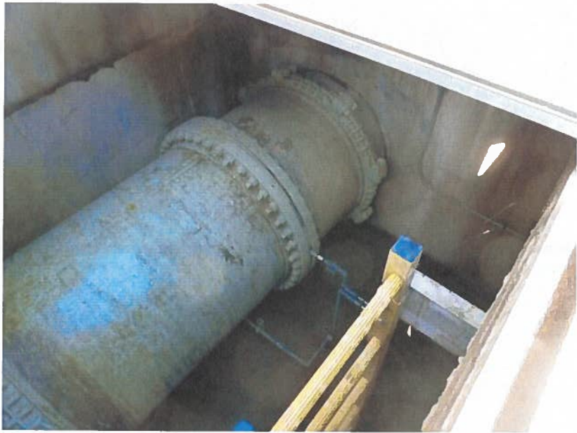
Photograph H –Pump Station Effluent Flow Meter
