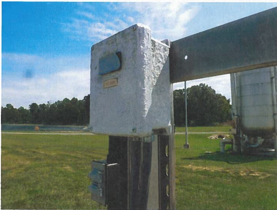
Photograph L – Influent Flow Meter Vault Instrument Display
