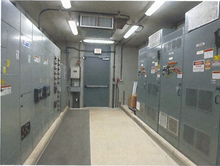
Photograph G – Pump Station Electrical Room
