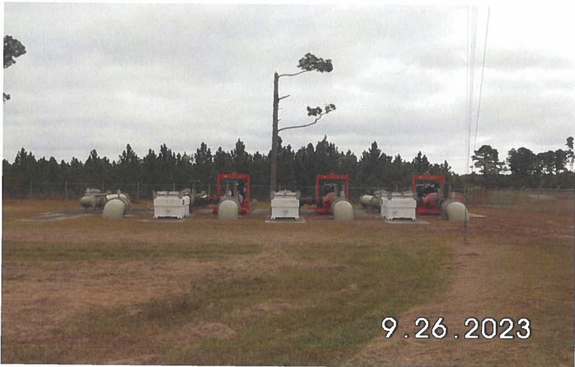
Photograph S – Interim Booster Station
