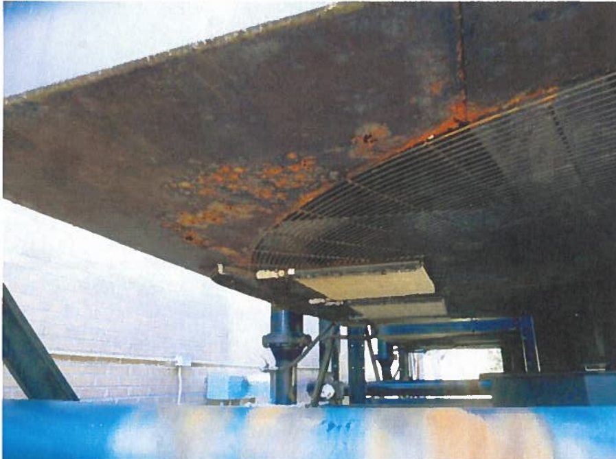
Photograph R – Corroded Radiator Fan Shroud
