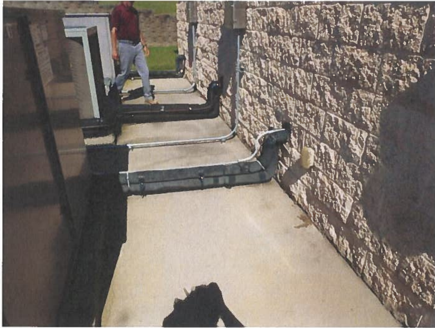
Photograph G – Failing HVAC Coolant Insulation
