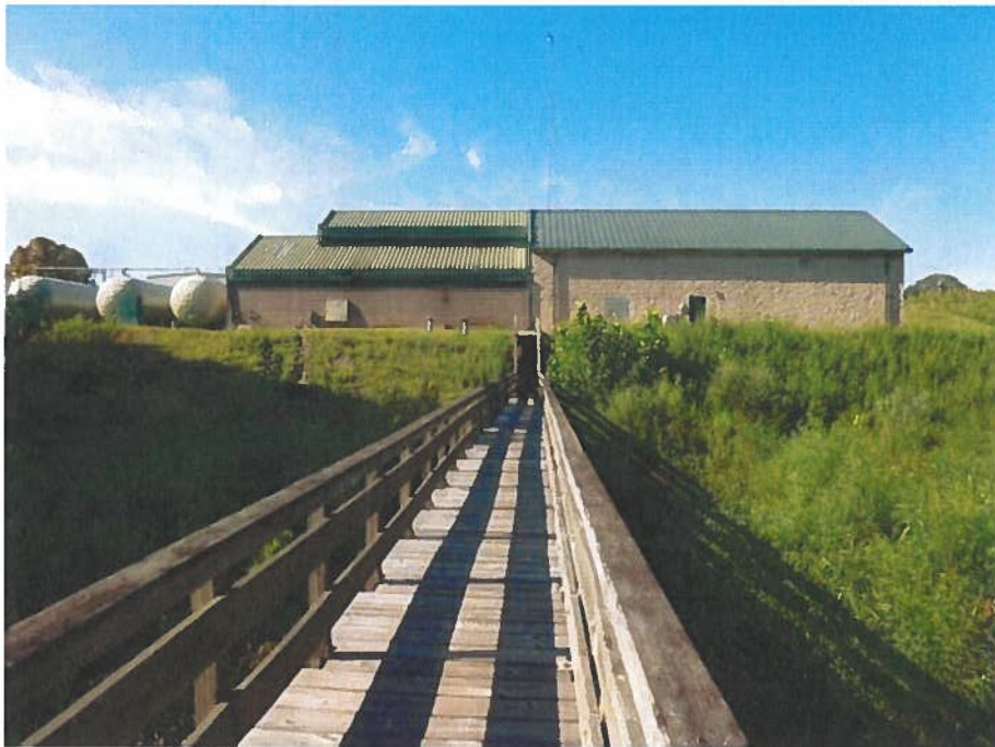
Photograph P – Distressed Air Backwash Pier Access
