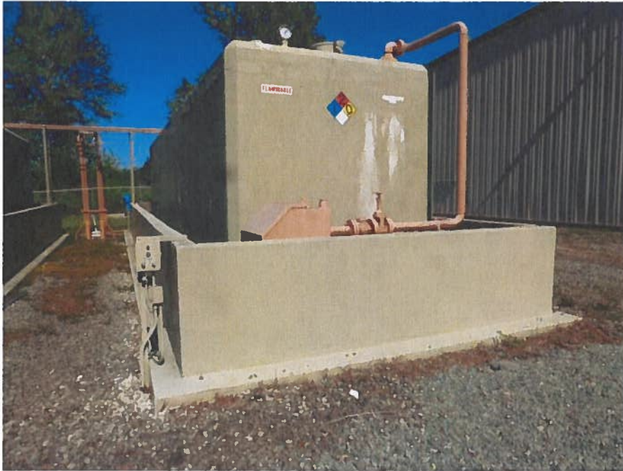
Photograph I – Diesel Storage Tank Efflorescence
