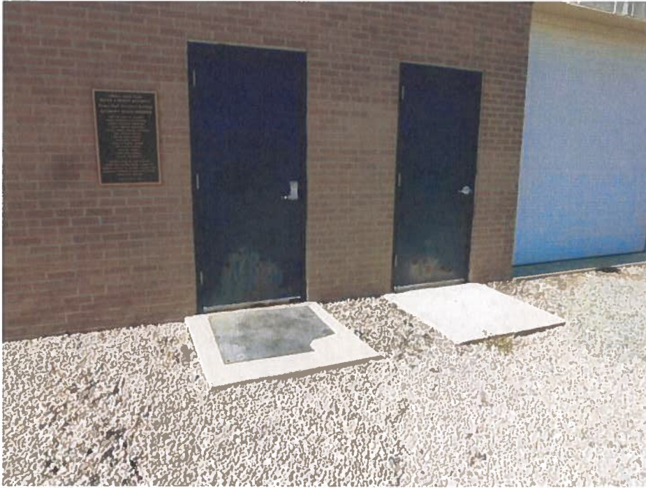
Photograph Q –Generator Building Corroded Doors
