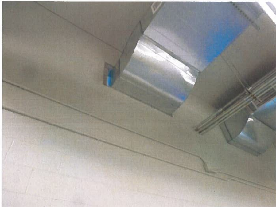
Photograph F -HVAC Penetration into Electrical Room
