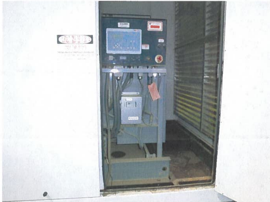
Photograph H – Influent Pump Station Generator Enclosure
