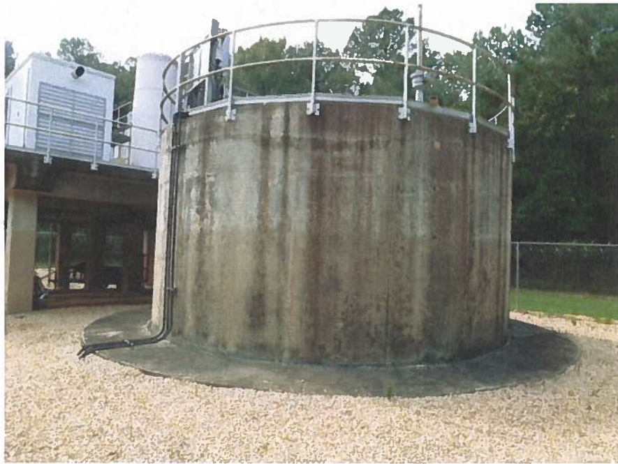
Photograph F - Raw Water Pump Station Wet Well
