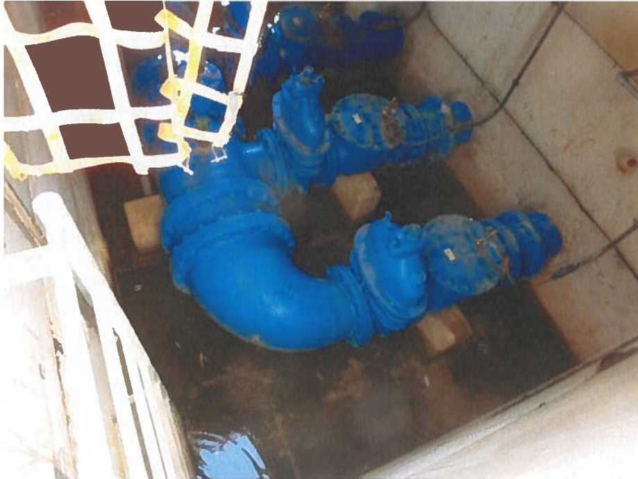
Photograph Q – Transfer Pump Station Valve Vault
