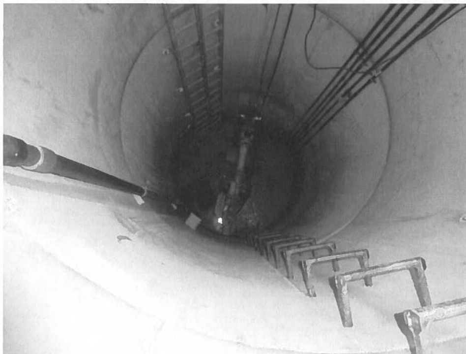
Photograph W –NPDES Meter Vault
