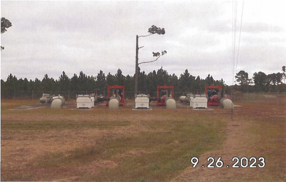
Photograph S – Interim Booster Station
