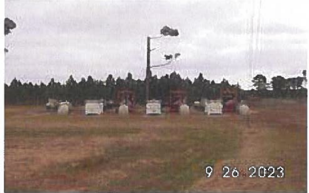
Interim Raw Water Booster Pump Station
