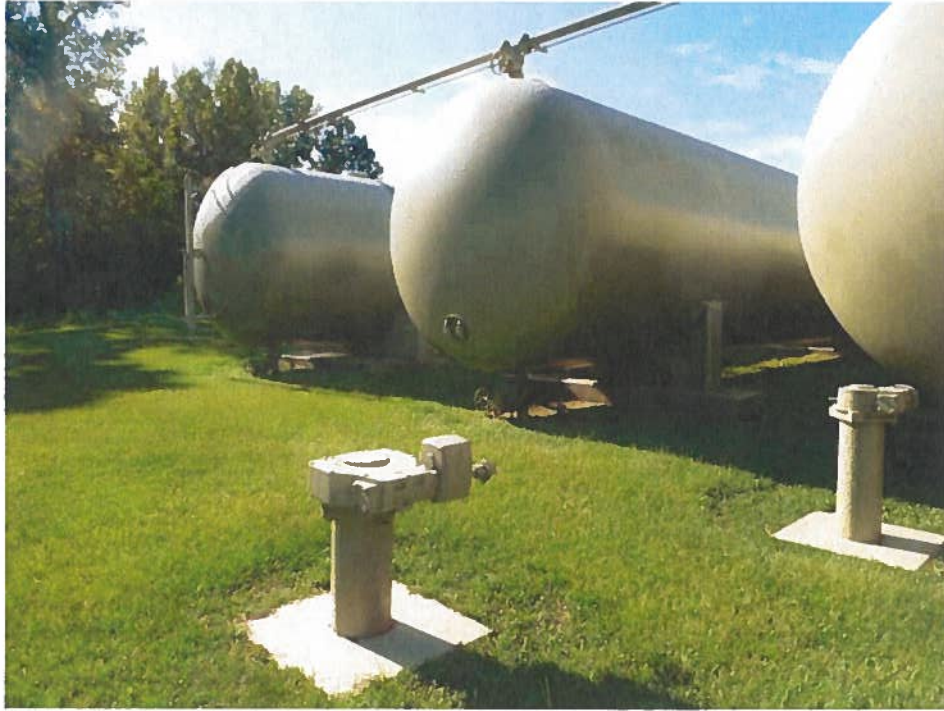
Photograph M- Surge Tank Valves Paint Peeling
