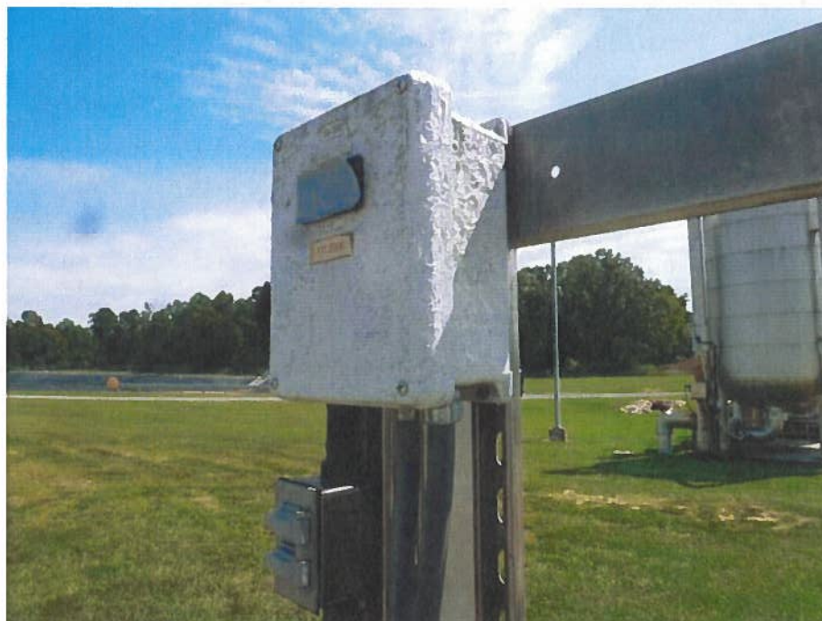
Photograph L – Influent Flow Meter Vault Instrument Display
