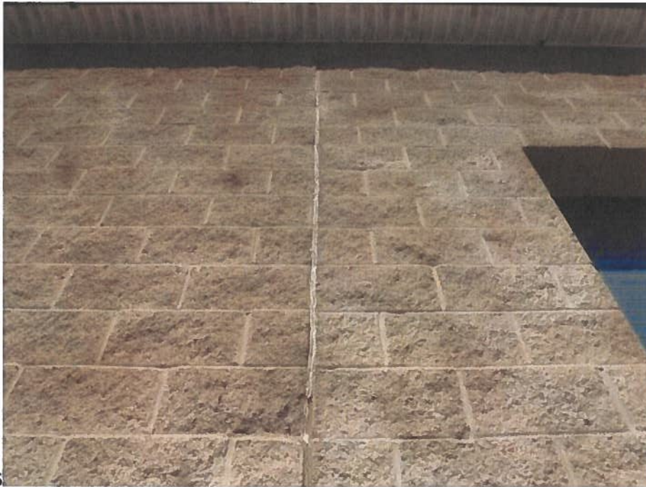
Photograph C – Existing Crack in Electrical Building Wall
