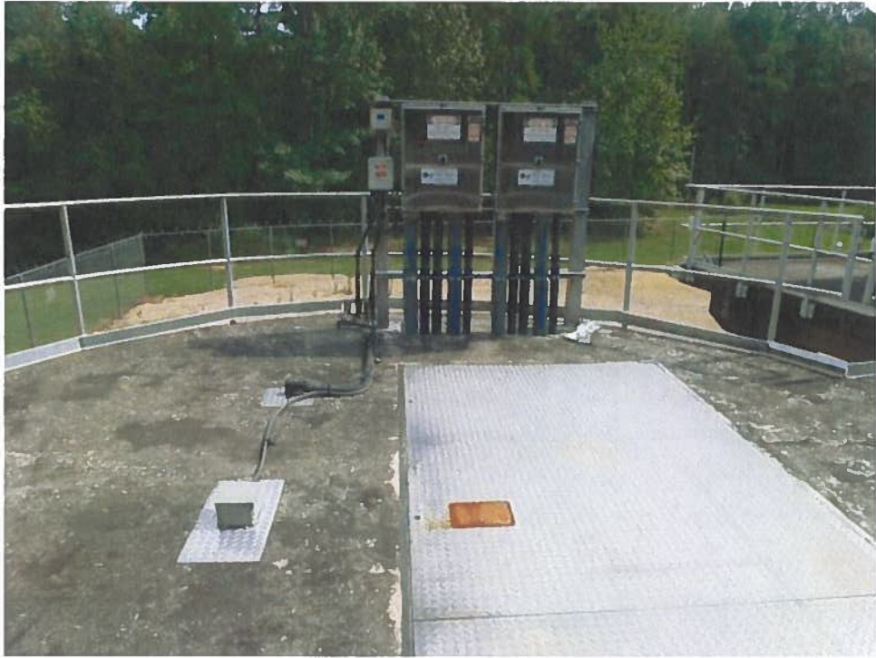
Photograph E – Raw Water Pump Station Level Display and Panels
