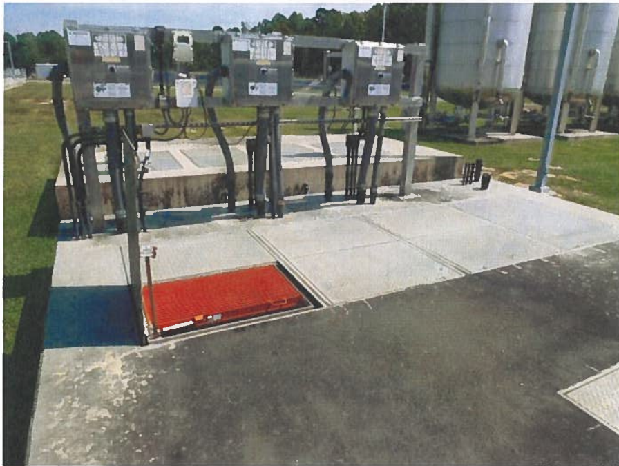
Photograph P – Transfer Pump Station
