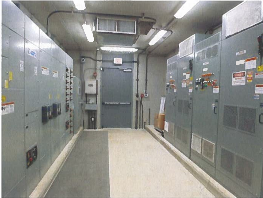
Photograph G – Pump Station Electrical Room
