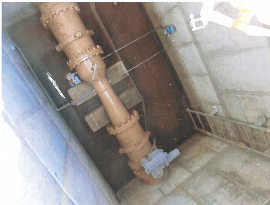
Photograph K -Influent Flow Meter Vault
