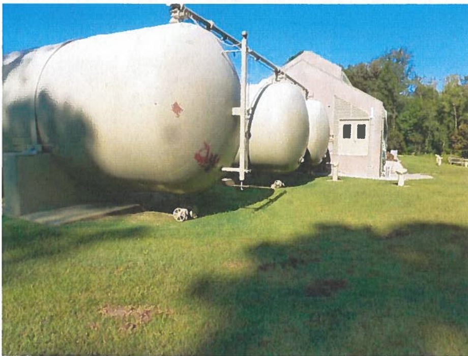
Photograph L- Surge Tank 3 Paint Peeling
