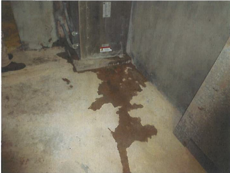
Photograph O – Filter Gallery Leak
