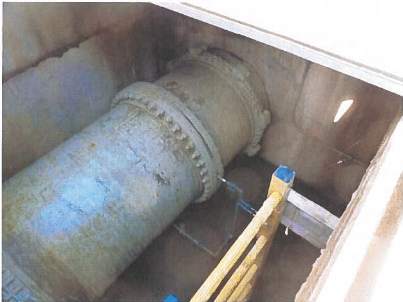
Photograph H – Pump Station Effluent Flow Meter
